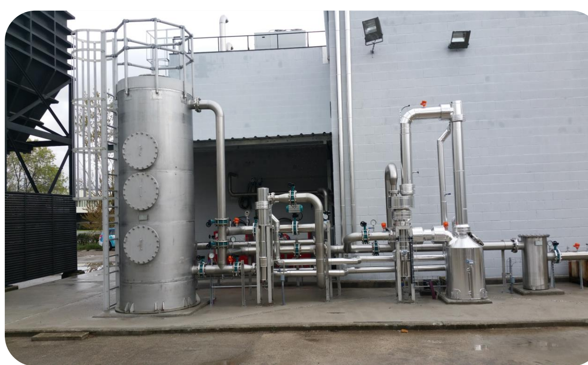
Figures 5. BTS-MPdry. Alcalá Oeste. WWTP made by BGasTech
